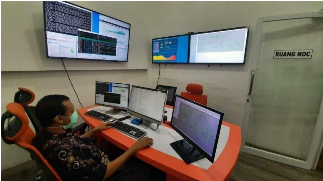
Gambar 2.9 Ruang Network Operation Center (NOC)
